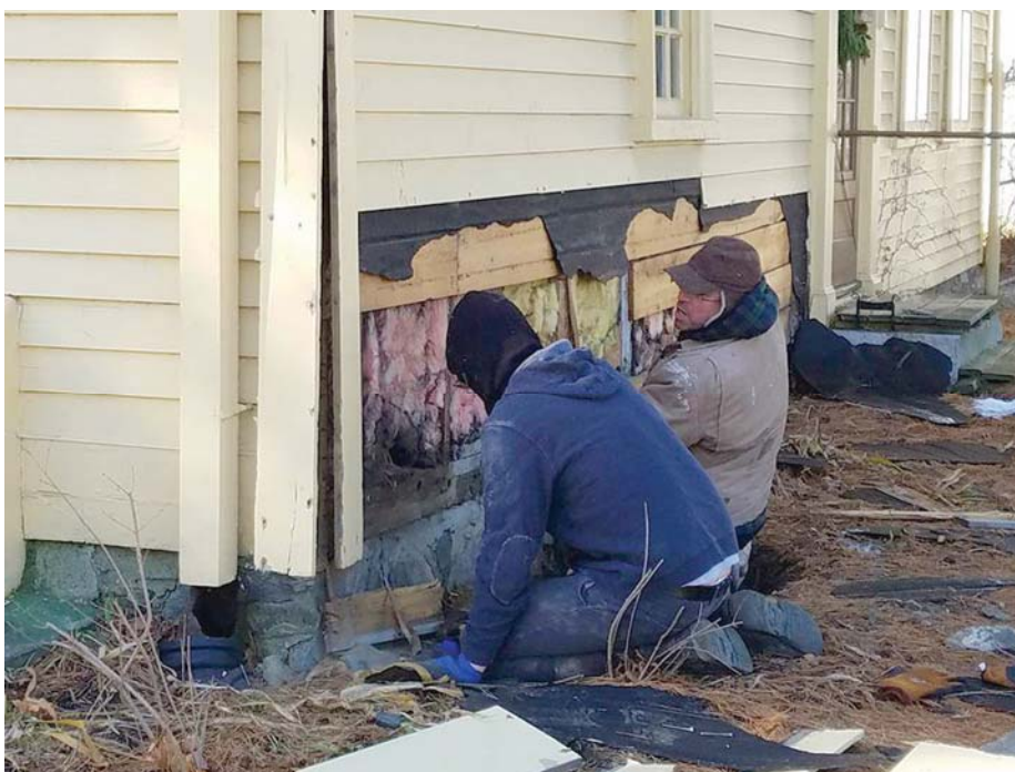
Workers removed clapboards and dug an exploratory trench on the north wall of the Jason Russell House to further examine structural problems. December 20, 2016.
